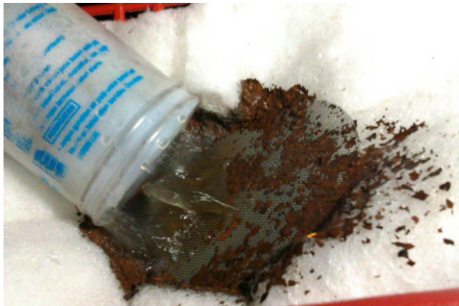
Scales mixed with rust at the flushing outlet
